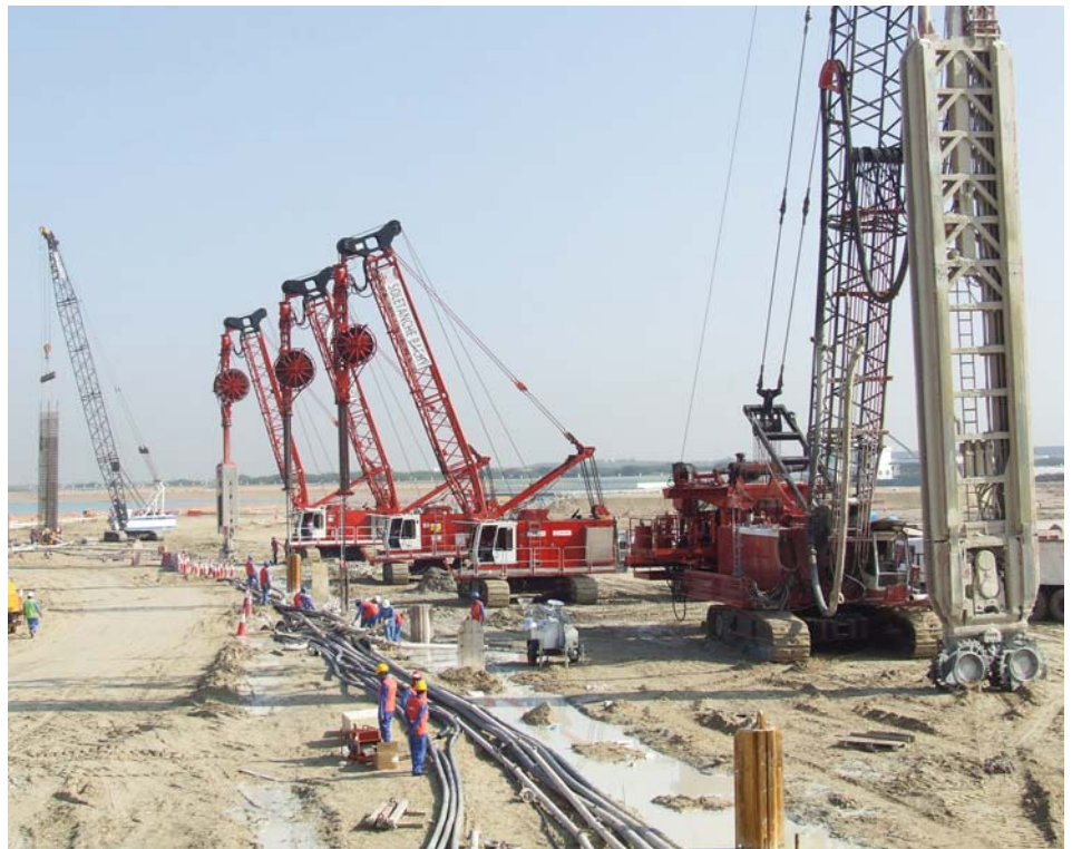
KS and hydrofraise along the future quay wall of Khor Al Raha
